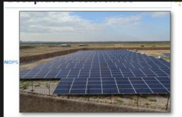
UNOPS 2017 Hybrid Power Generation Facility
