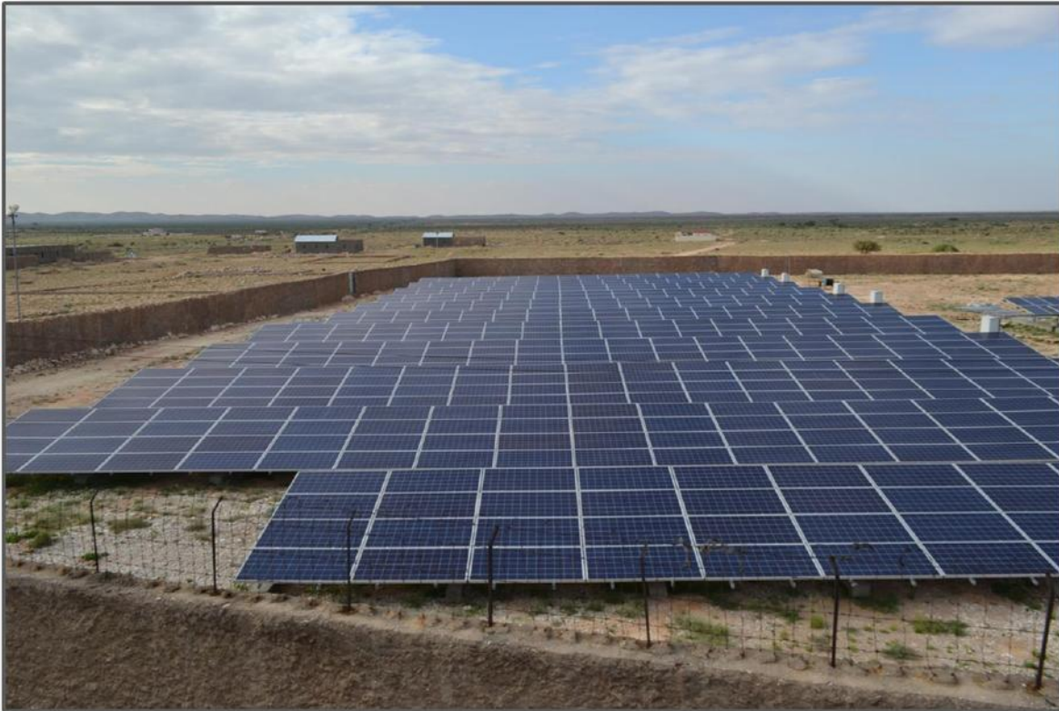
Hybrid Power Generation Facility 2017
